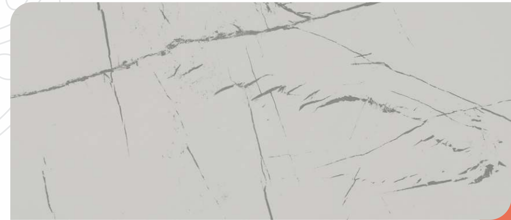
8005 B-103 | STOMY CRACK
